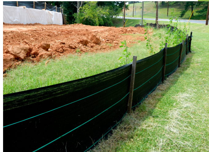
Keep your silt fence up and you'll be fine! Photo via Canva.
